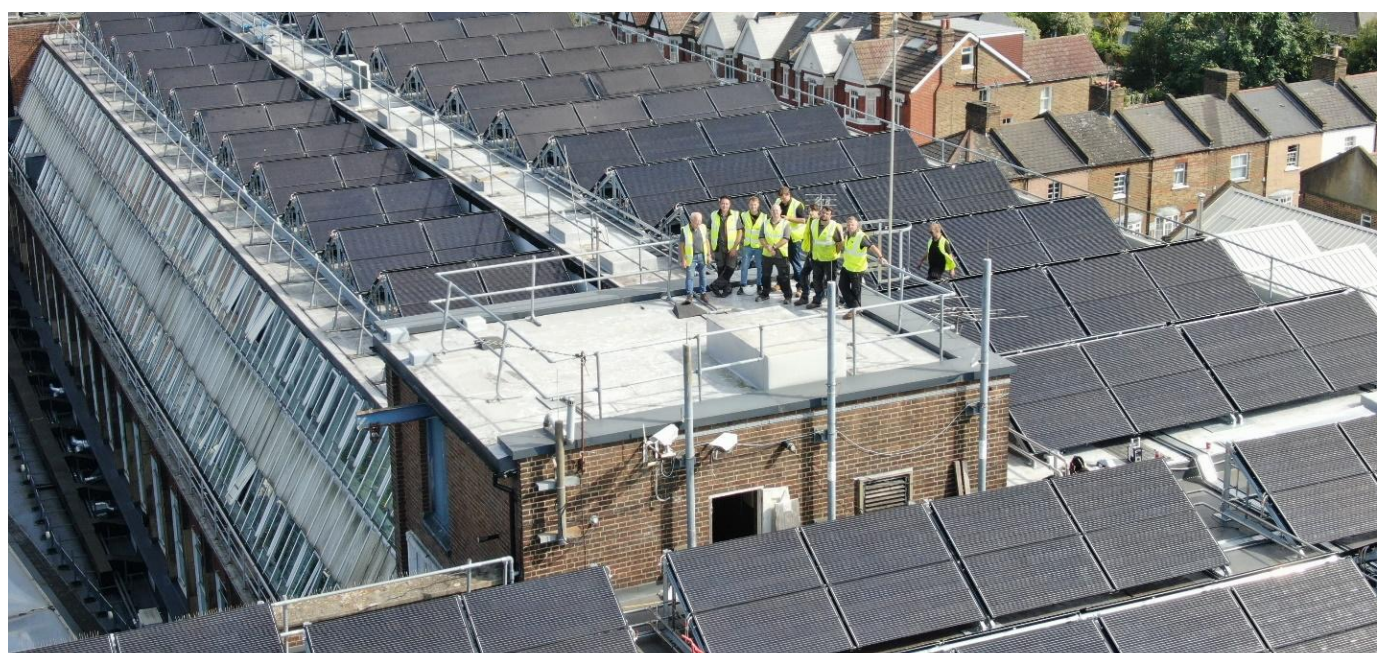
Image: Solar-PVT installation on the roof of the Ealing Campus, University of West London
