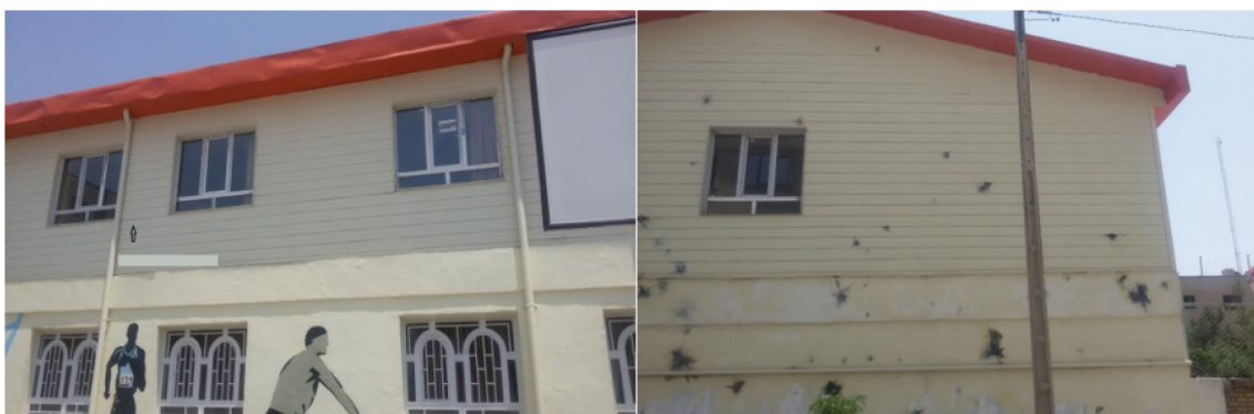
Figure 8. Dry facades problems in LSF system: right panel: striking some heavy things to dry facades. Left panel: bad performance of construction or insulation.
