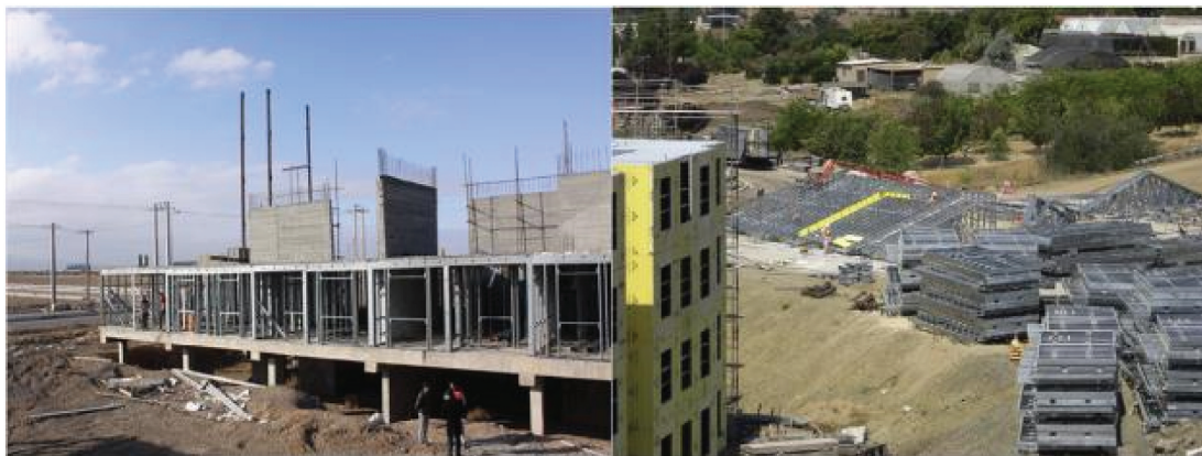
Figure 5. Left panel: Combination of LSF system with shear wall in a 7-story school. Right panel: panelization in LSF buildings (Yu 2016).
