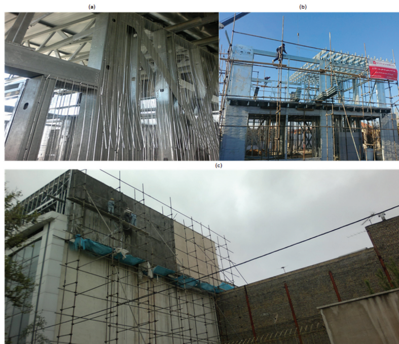
Figure 13. Panel (a) and (b): Screwing expanded metal lath on studs and runners. Panel (c): Covering white mortar cement on the metal lath.
