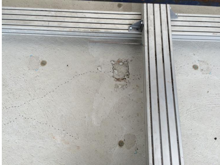
Figure 4: Slab centre loading visible punching shear failure together with crack pattern.
