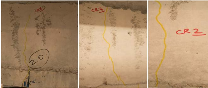
Figure 2. Detected cracks on body of the BGB in damaged state.
