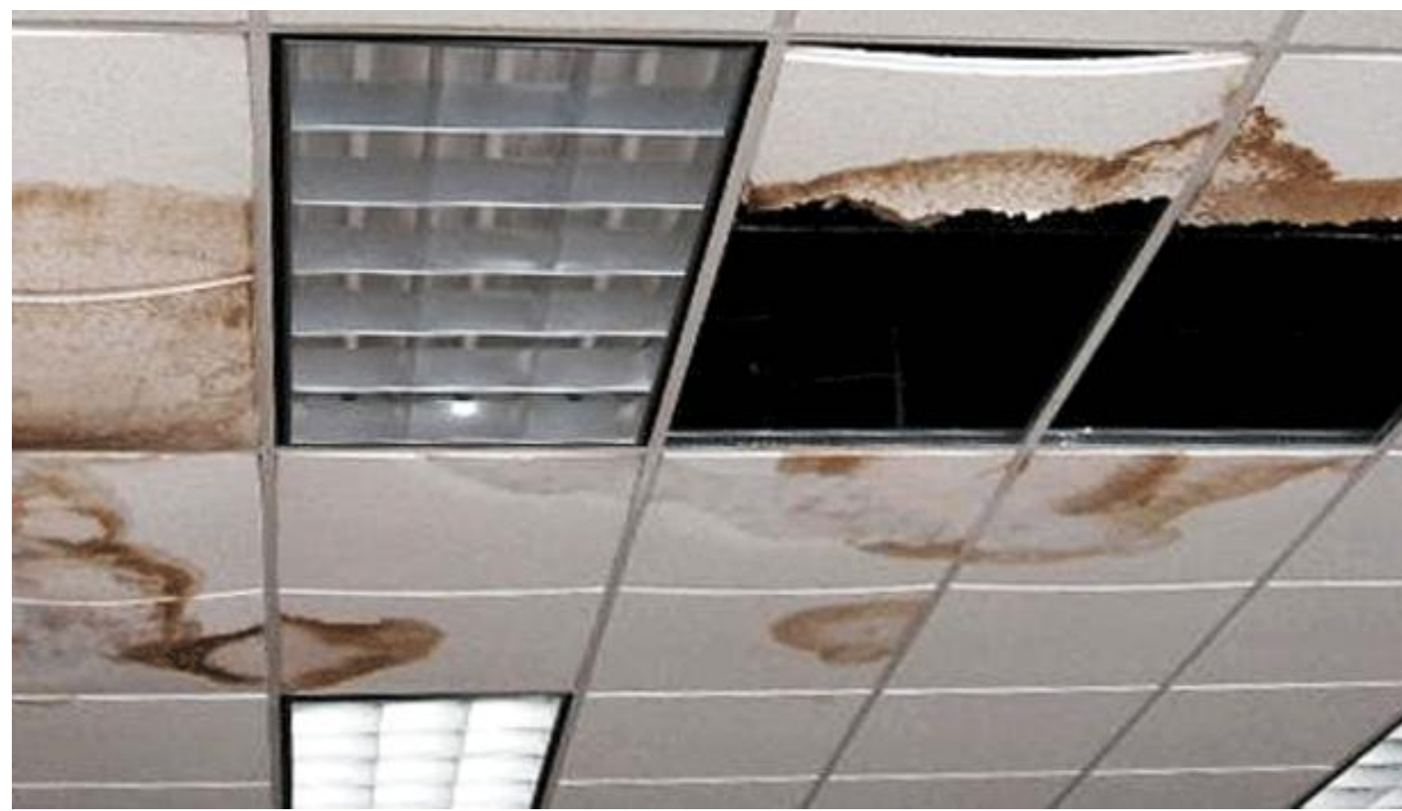
Figure 1 – Leak damaged ceiling tiles
