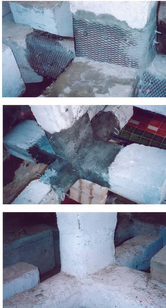
Fig. 6. Fabrication details, inserting expanded wire mesh layers and rendering them with mortar to make ferrocement layers.
