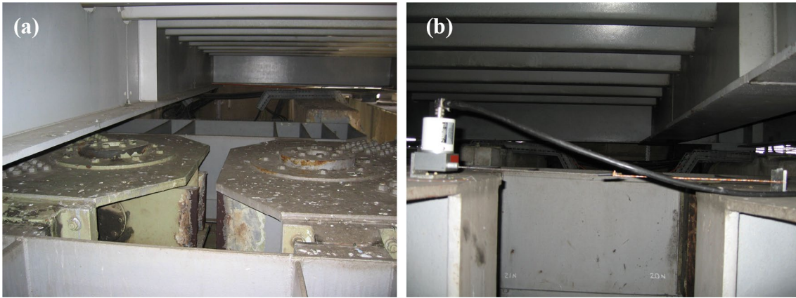
Fig. 5 New bearings at the Saltash tower (a) and setup of string gauge for measurement of the expansion joint thermal dilation (b)
