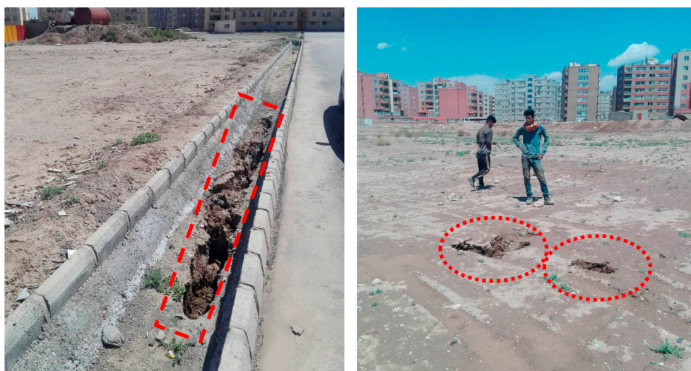
Figure 16. Evidence of qanat outlets collapse and related surface damage at the investigated site.
