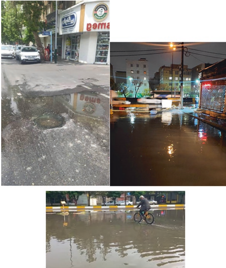
Fig. 8.2 Examples of UDIs' failures in Tehran, Iran
