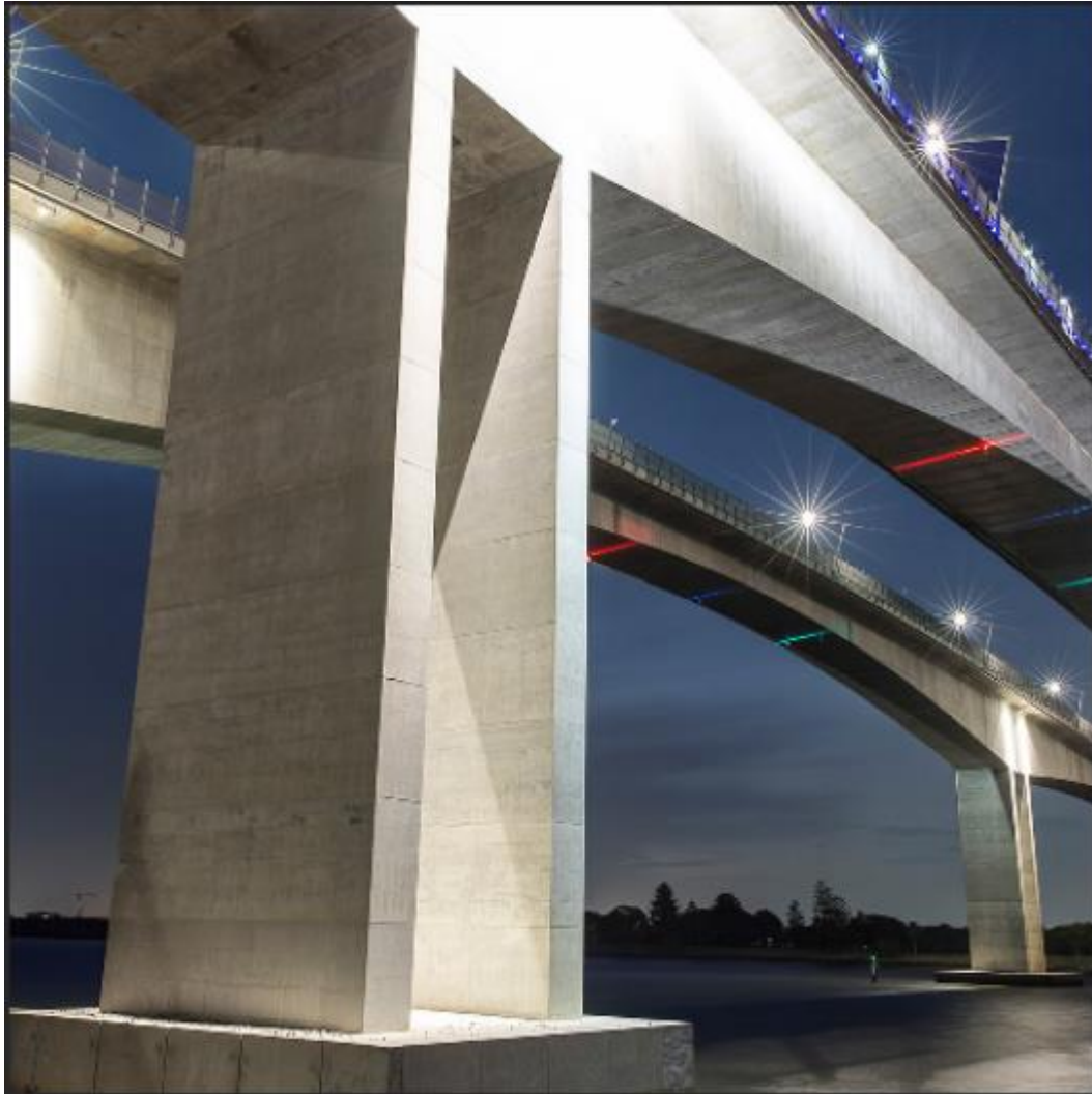
Figure 2.16 Gatwick bridge in Austria (Stainlessrebar, 2021)
