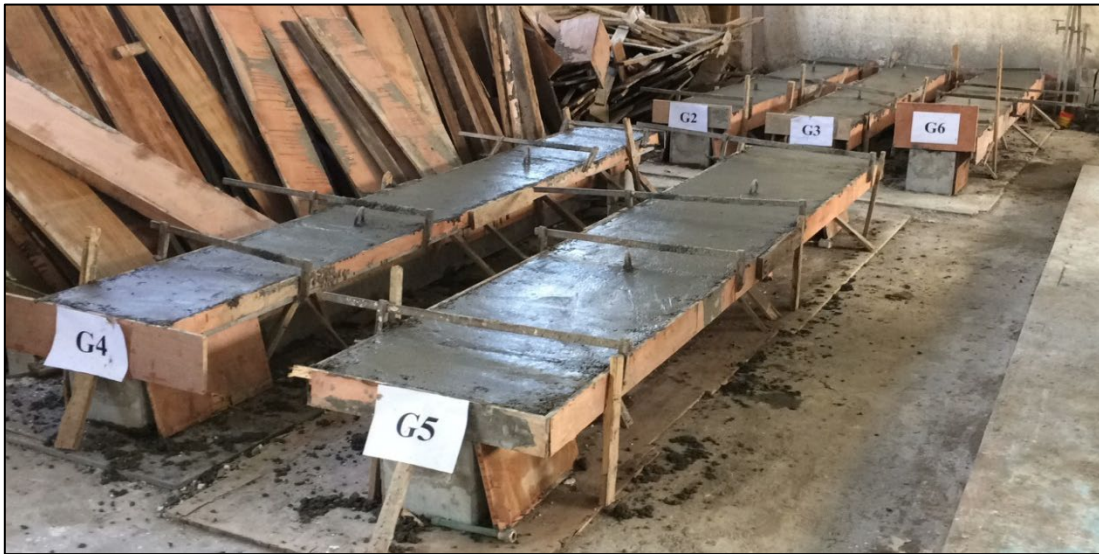
Figure 15: Finishing casting concrete for the rest of topping slab (G2 to G6)
