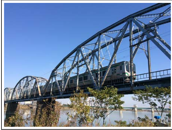
Figure 5. Polarimetric FastGB SAR-R system set up beside metallic railway bridge while a train passes.
