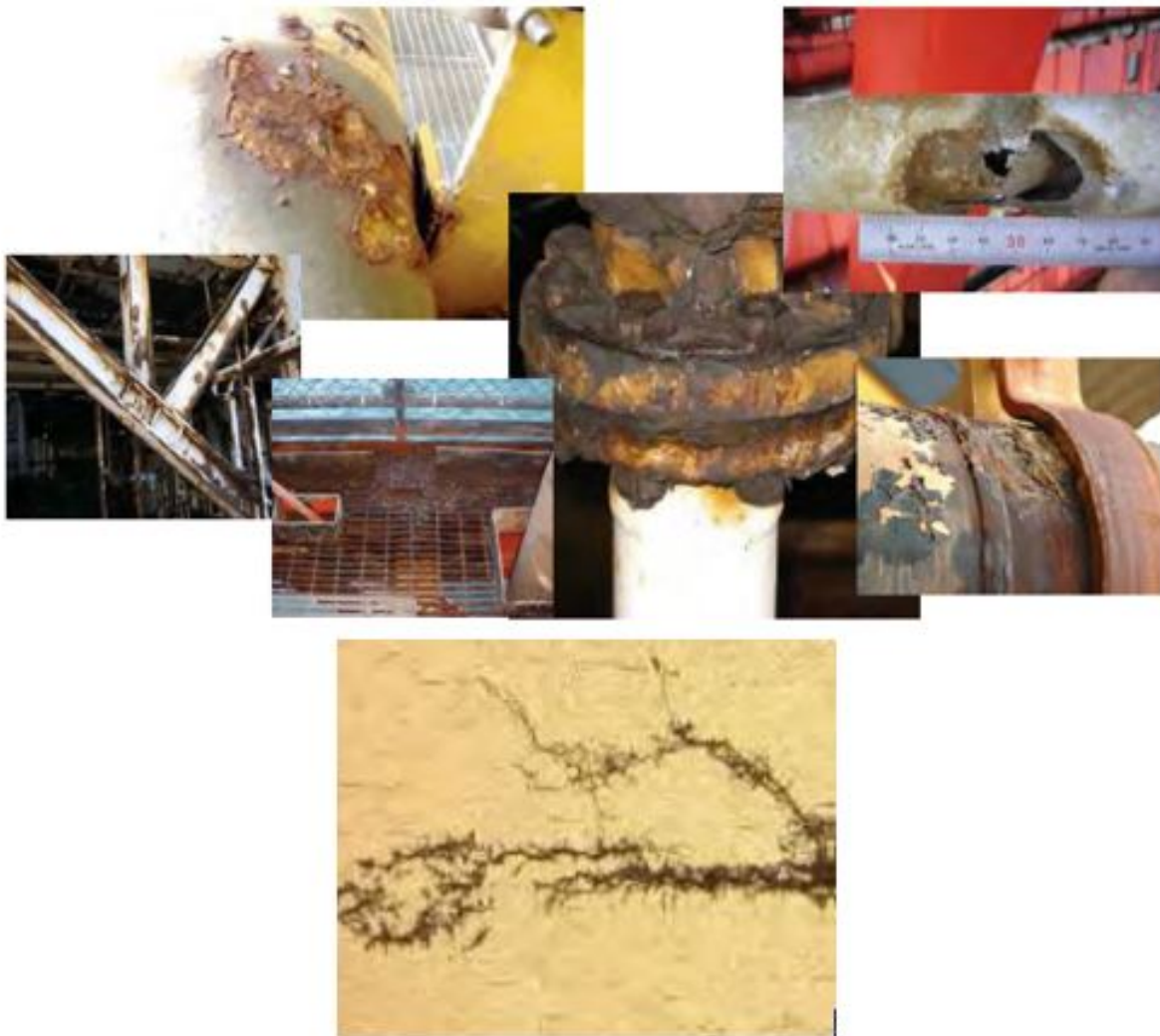
Figure 2.3: Corrosion on gratings and Cracks on plates of Offshore structures [4]
