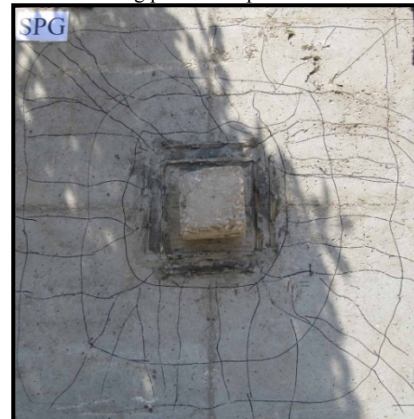
Cracking pattern of specimen SPG
