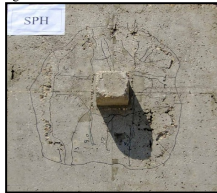
Cracking pattern of reference specimen SPH
