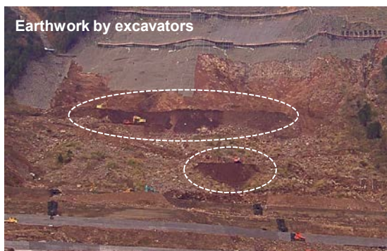
Fig. 12. The areas introducing differential phase after the earthwork due to the wind-driven soil erosion indicated by white dash circles.
